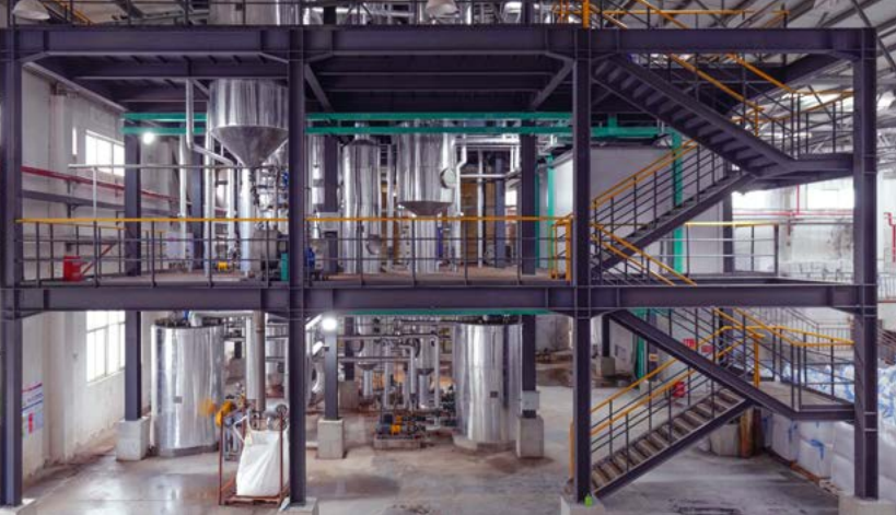
The new fully automated waste water desalination plant in Donghai
