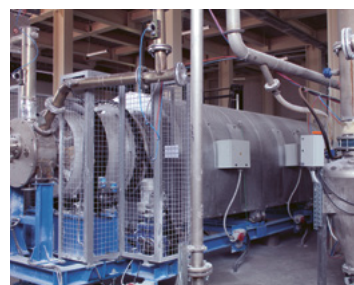
The new calcining plant at the Zvornik site
